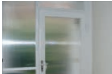
Many doors don't close as tightly as they appear at first glance
